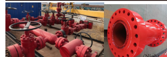
MANIFOLDS - DRILLING & SPACER SPOOL
